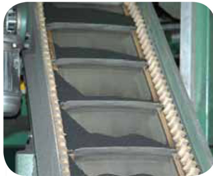
FRG - 3 Chemical powder conveying
